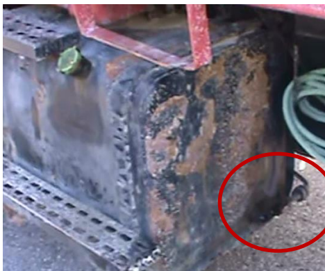
Fuel leak at connection
