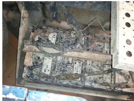
No protective cover on batteries
